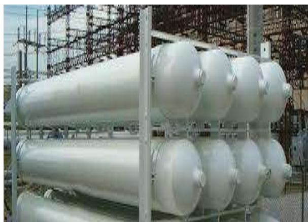
Fig 7: Cylinders for Hydrogen Storage
