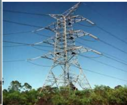
Fig. Self supporting tower
