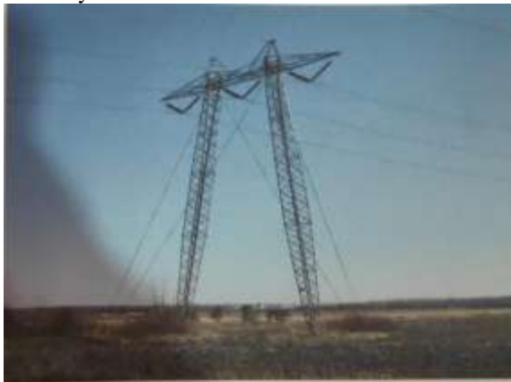
Fig. Guyed tower
