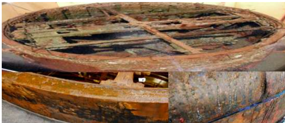
Fig. 1: Shows typical turret system corrosion failure (Courtesy: metallurgical technologies, 2015)
