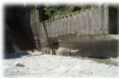
Photograph 4 Damaged Training wall
