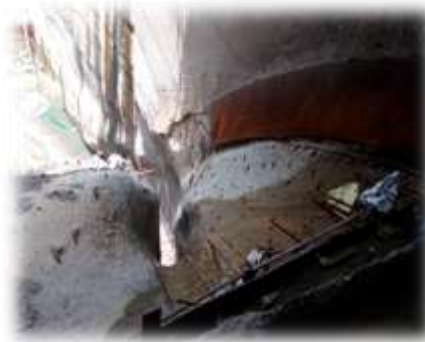
Photograph 2: Damages in Spillway Bay no 1
