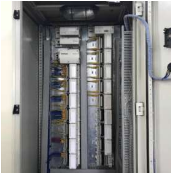
Figure 10: AC800M controller in boiler level control system
