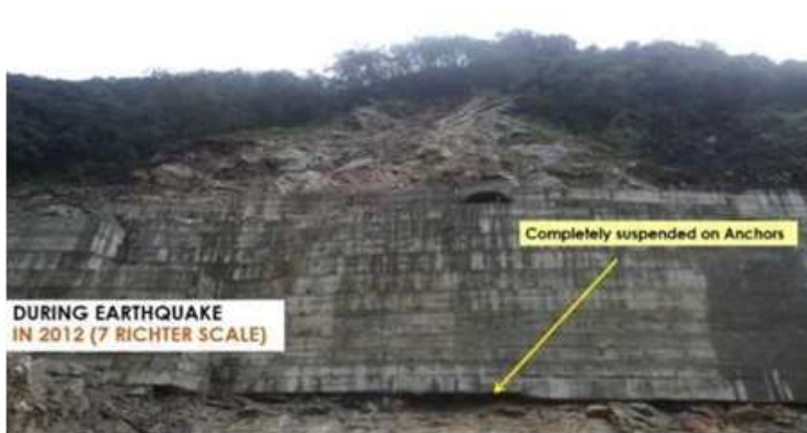
Figure 17: Condition of stabilized slope with pre-stressed anchor after 2012, earthquake (Magnitude 7)
