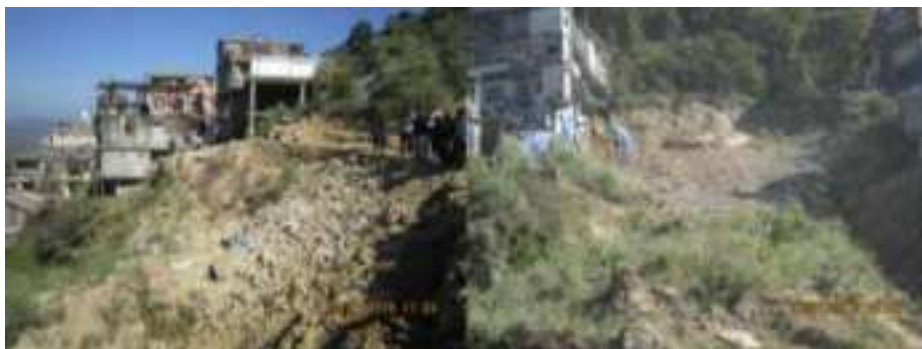
Fig. 2: Road collapsed due to continuous erosion at valley side
