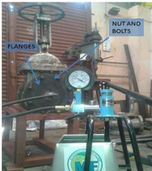
Fig 1.1:- Present condition of hydro test
