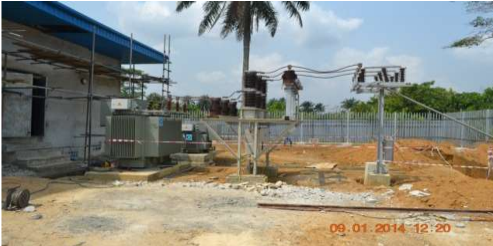
Plate.4: 33kva Electricity Supply
