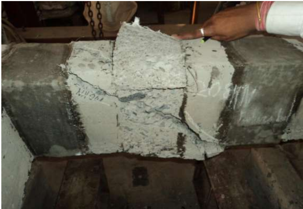
Figure 14 shows the failure pattern of the retrofitted beam, when the GFRP sheet was removed.
